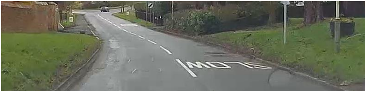
R3.7 - Condition score 0 - for centre Lines and Folly Bank Junction Markings
