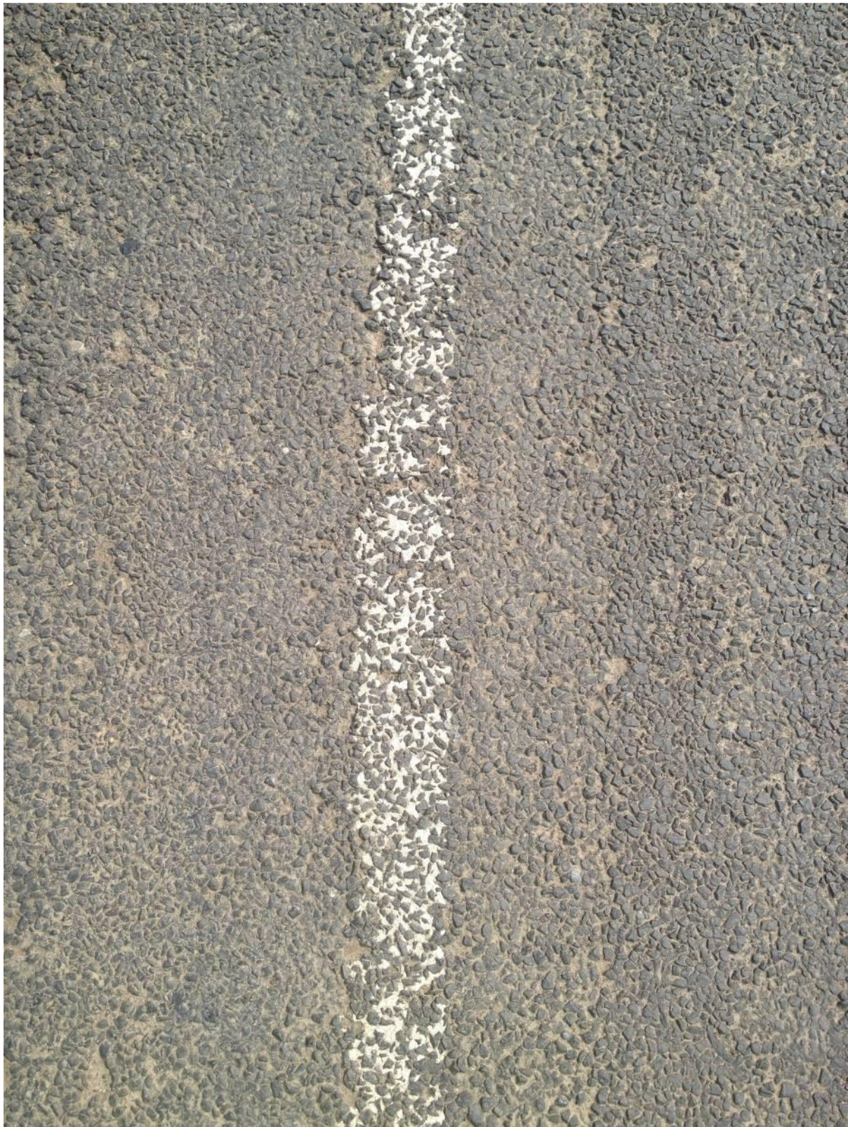
Figure C.11 Condition score 10 – close-up
