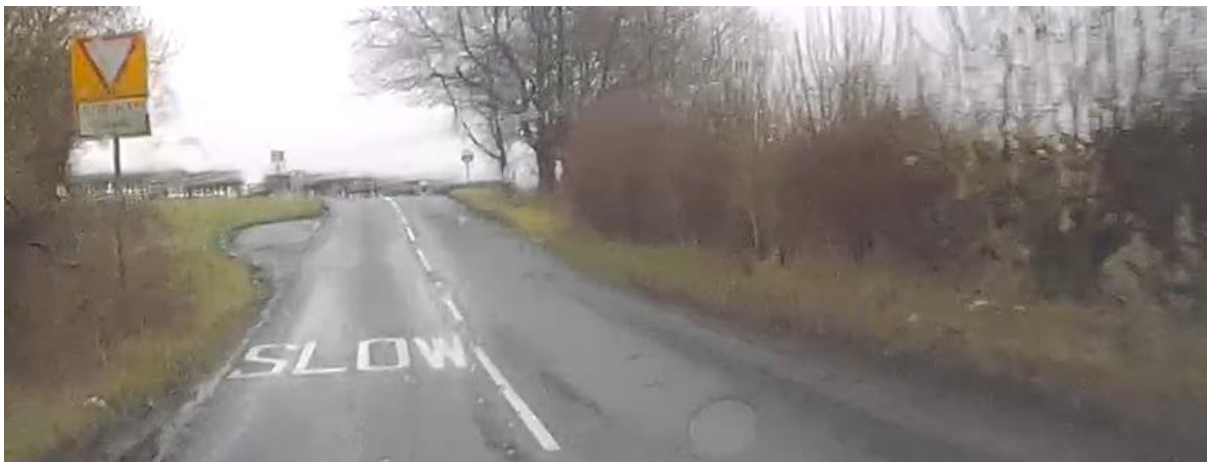
R5.26 - Condition Score 40 (Junction markings)
