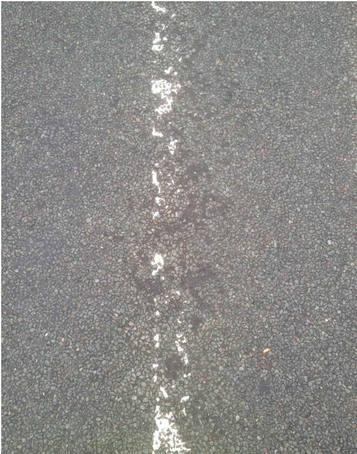
Figure C.13 Condition score 0 – close-up
